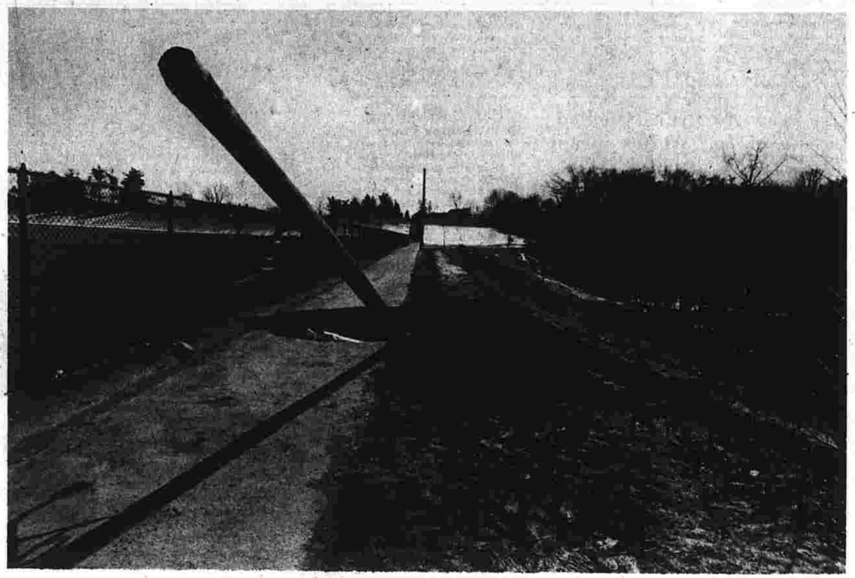
Hole Where the Walkway Was Recent heavy rains and a leak in an underground conduit next to Memorial Field at Manchester High School combined to wash out this substantial area outside fence on the west side of the field. The conduit is part of a system for removing surface water from the field and feeding it into Bigelow Brook. According to Charles Crocinni, assistant superintendent of buildings and grounds with the Board of Education, the pipe will be repaired and the area rebuilt by the town highway department. The pole, which lights the path leading to the tennis courts on Center St., will have to be reset, Crocinni says. The repairs will probably be completed by the end of the week, according to Crocinni. (Herald photo by Pinto)
